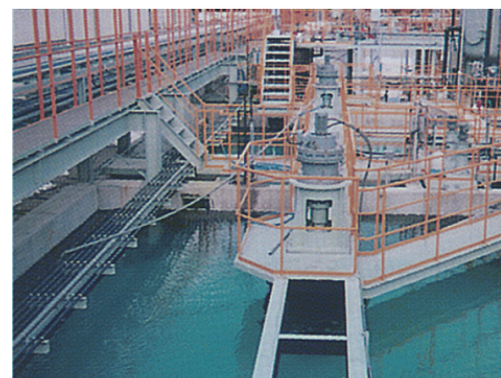
Wastewater Treatment Equipment
