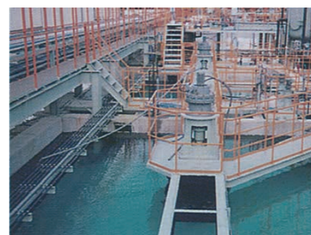
Wastewater Treatment Equipment
