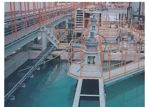
Wastewater Treatment Equipment
